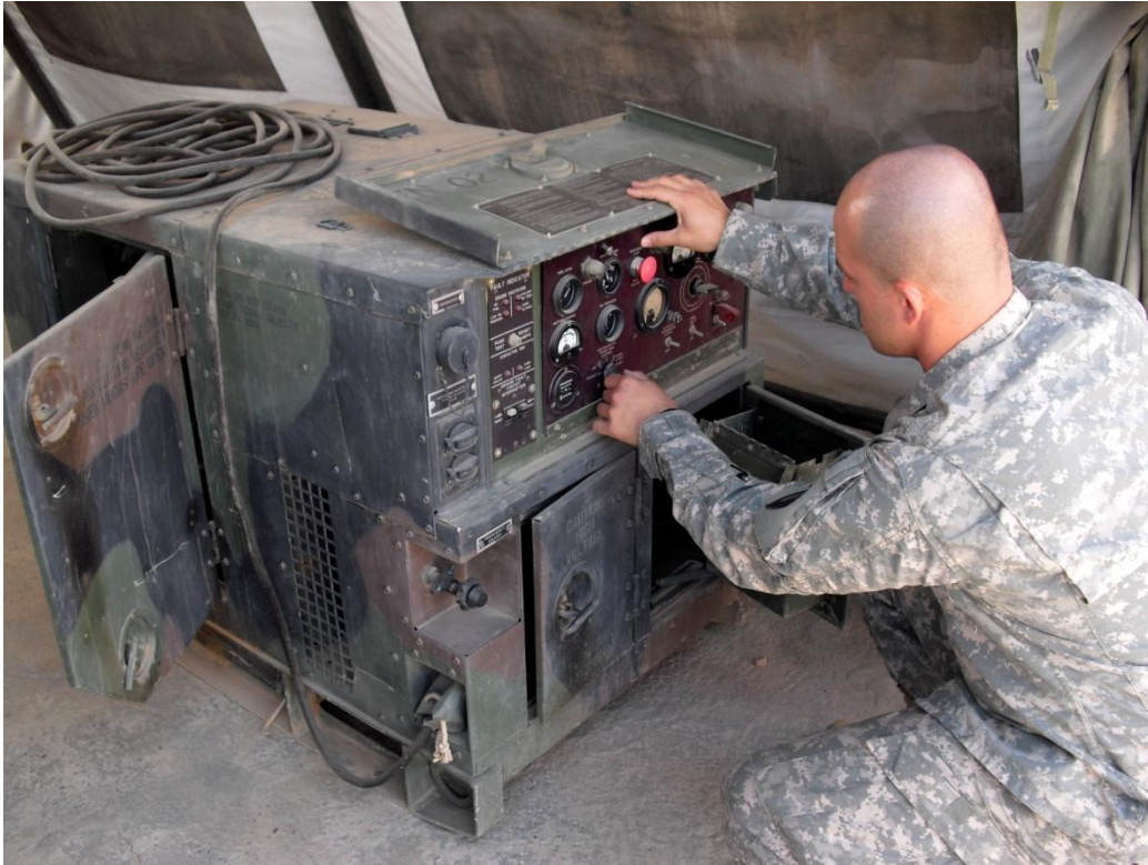
Spc. Juan Nieves, a power generation mechanic with the 271st Human Resources Company, with the Special Troops Battalion, 96th Sustainment Brigade, and a native of Maricao, Puerto Rico, is conducting a Preventive Maintenance Check Service on a Generator set 5KW.
